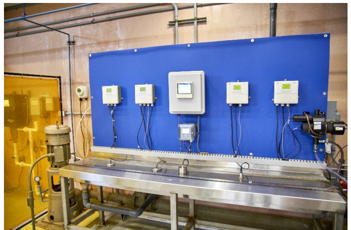
Standard configuration for online monitoring equipment instrument bench at our facilities
